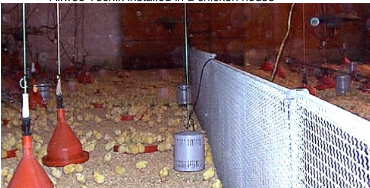
Airfree Technik installed in a chicken house
